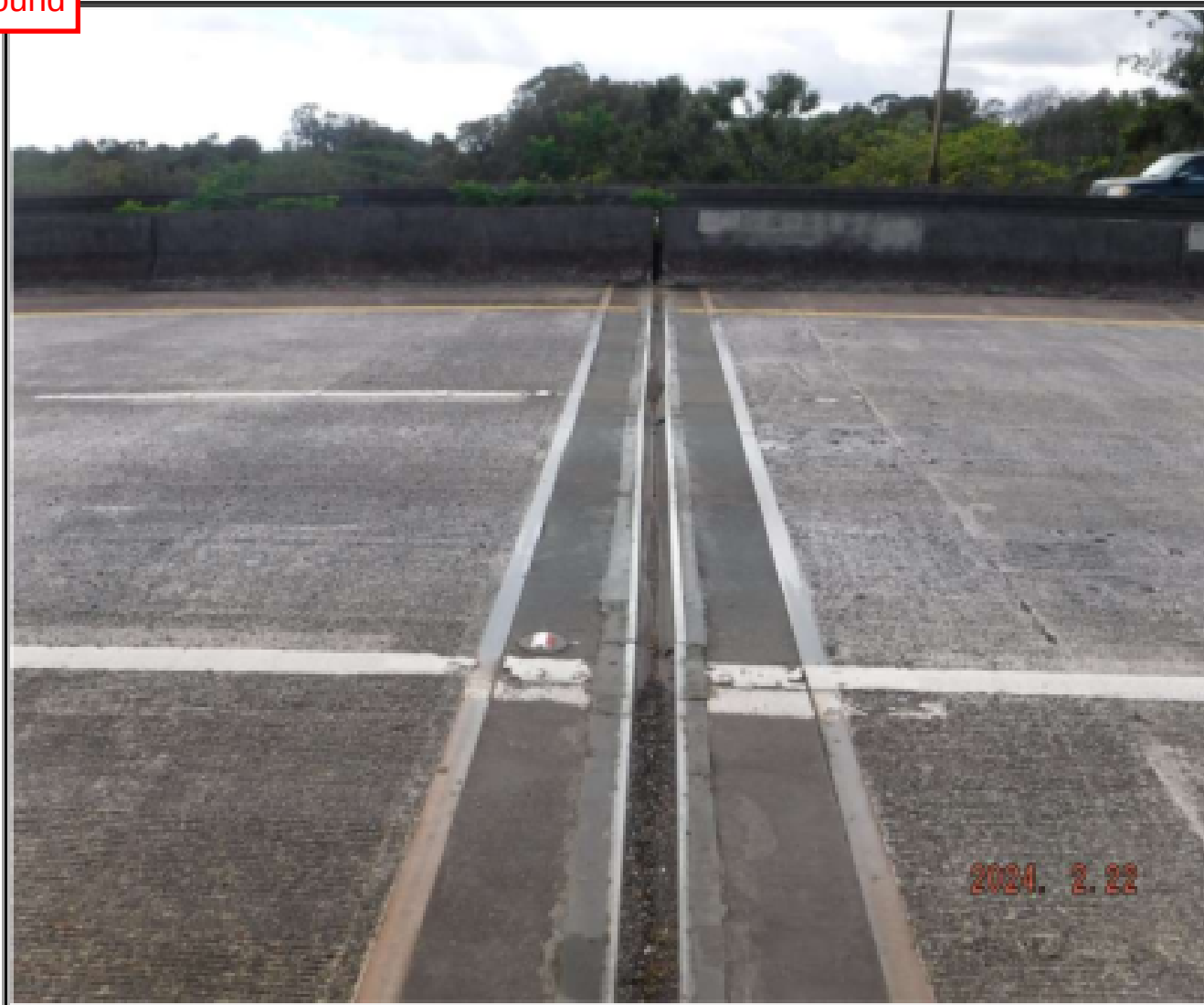
Photo 16. Expansion joint, S4, both lanes, P3 @ 55', looking west. Minor debris impaction throughout, CS2.
